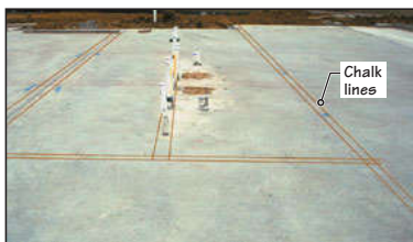
FIGURE 4 Chalk lines on the slab indicate the location of the walls. Note that plumbing pipes align and are located within the thickness of the wall.
